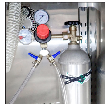
FIG. 9. Always strap the CO 2 cylinder into the cabinet.
