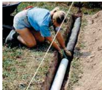
Figure 275: Underground Refrigerant Piping.
