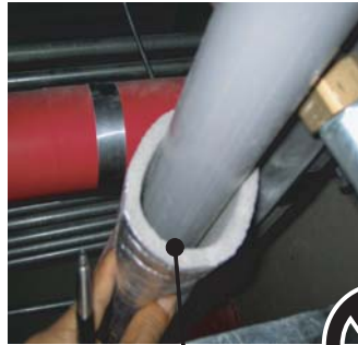
Loose fitting wrong insulation
