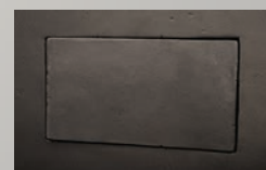
CONCEALED CONTROL PANEL
