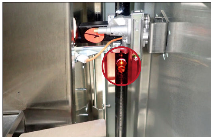
Fig. 1. Pressure testing port located near the leftmost burner.
