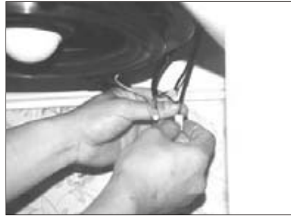
12. Connect both wires (blk) on hood to either power supply (blk or wht). Ground green wire.**
