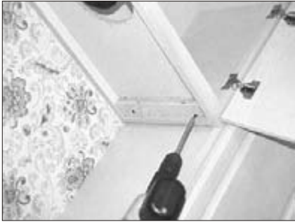
5. Reinforce cabinet base with 1x2 wood strips if additional strengthening is required. Unscrew and remove bottom grease splash shield.
